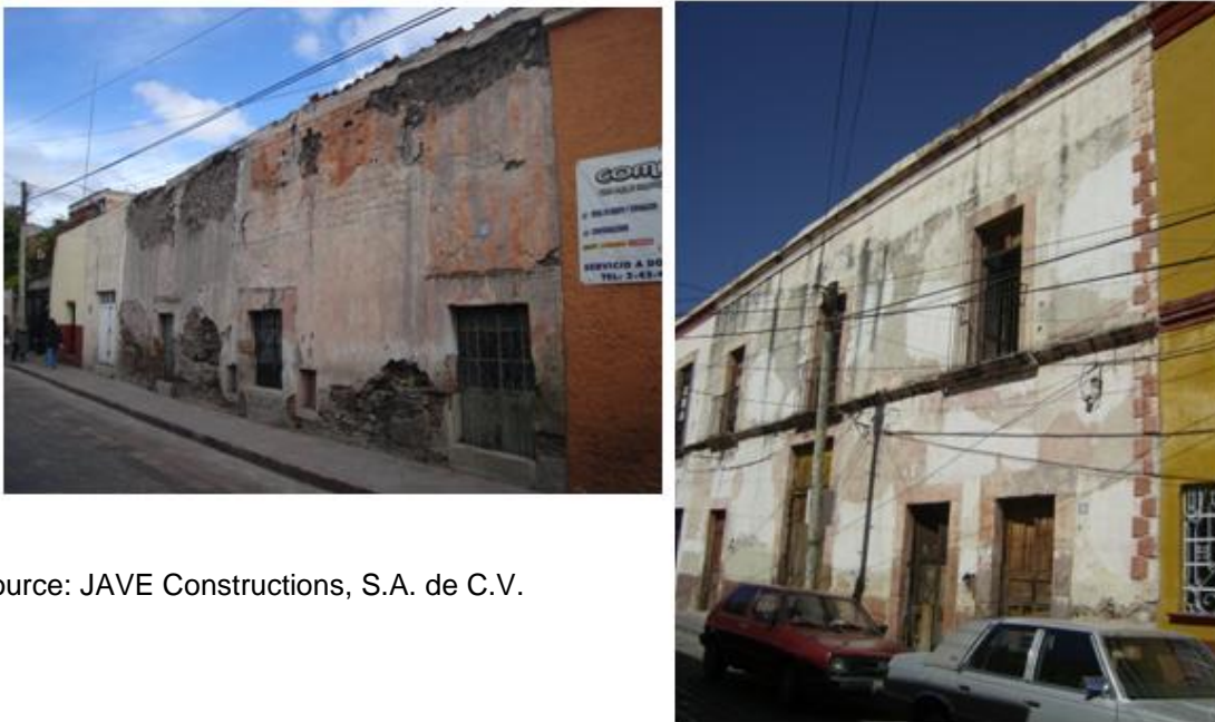
Figure II.25 Examples of abandoned and ruined heritage buildings located at 55 Nicolás Campa South (left) and 20 Mariano Escobedo (right)
